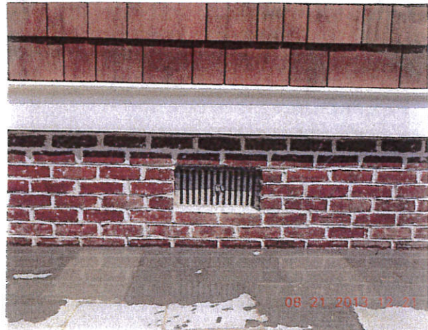
LOUVERED VENT - TYPICAL OF 2
